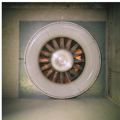
Application de ventilation
